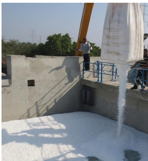
Tanks being loaded with 30 % fill fraction of ActiveCell® media
