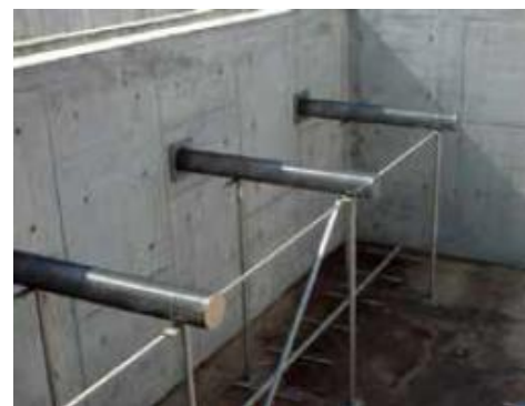
Effluent Screens and Aeration Grid
